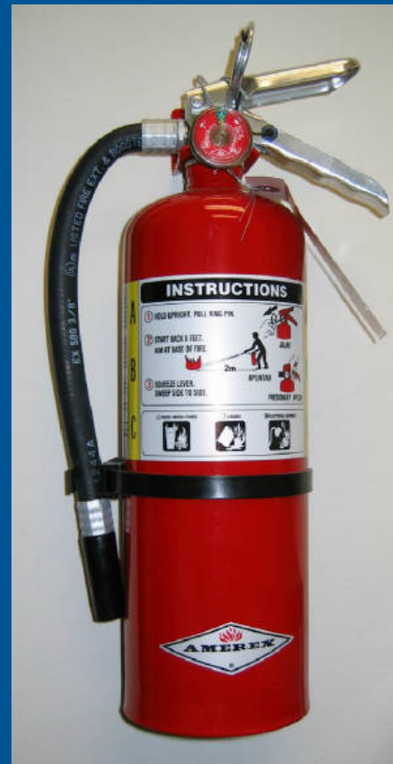
Combination Fire Extinguisher
