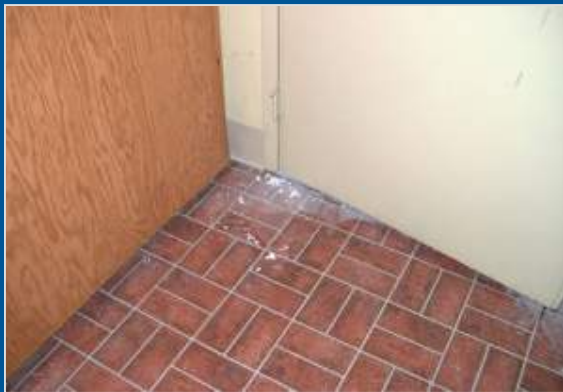
Asbestos debris on floor
