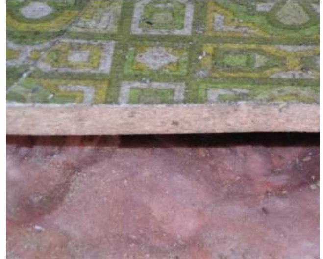
Sheet vinyl containing asbestos
