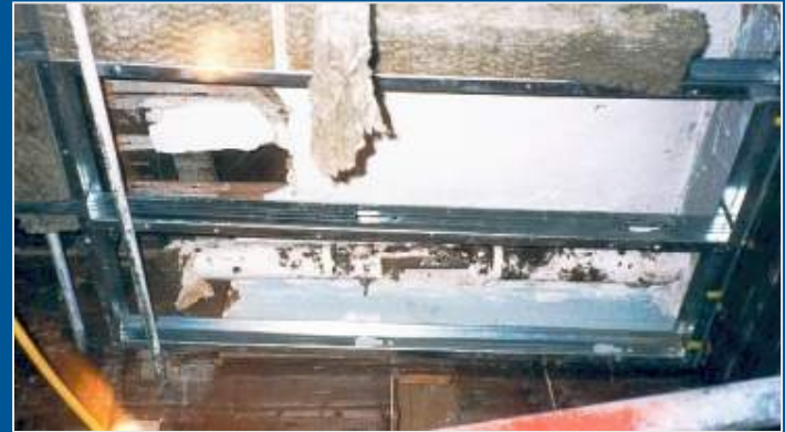
Damaged asbestos pipe insulation
