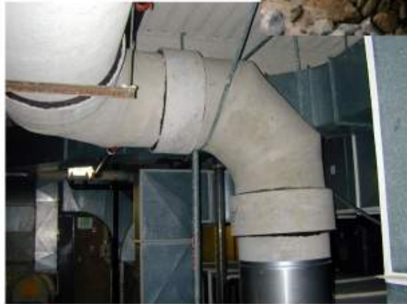
ASBESTOS CEMENT LAB FUME HOOD EXHAUST DUCT
