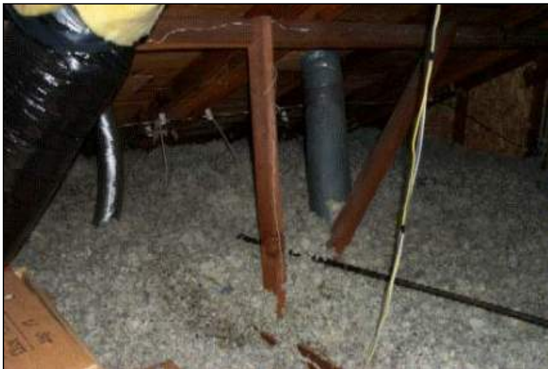
Vermiculite insulation in attics
