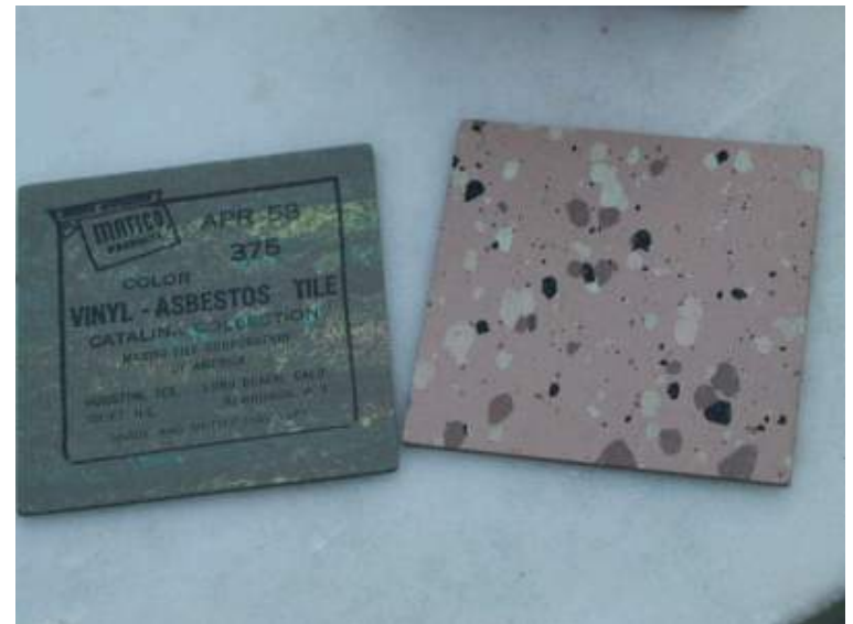
Vinyl asbestos flooring
